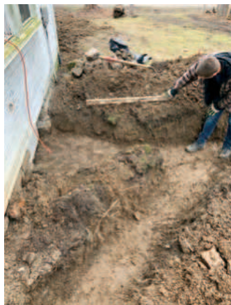
To keep water away from the foundation, we installed 300 feet of drain tile. Patrick Morrissey checks the slope.
